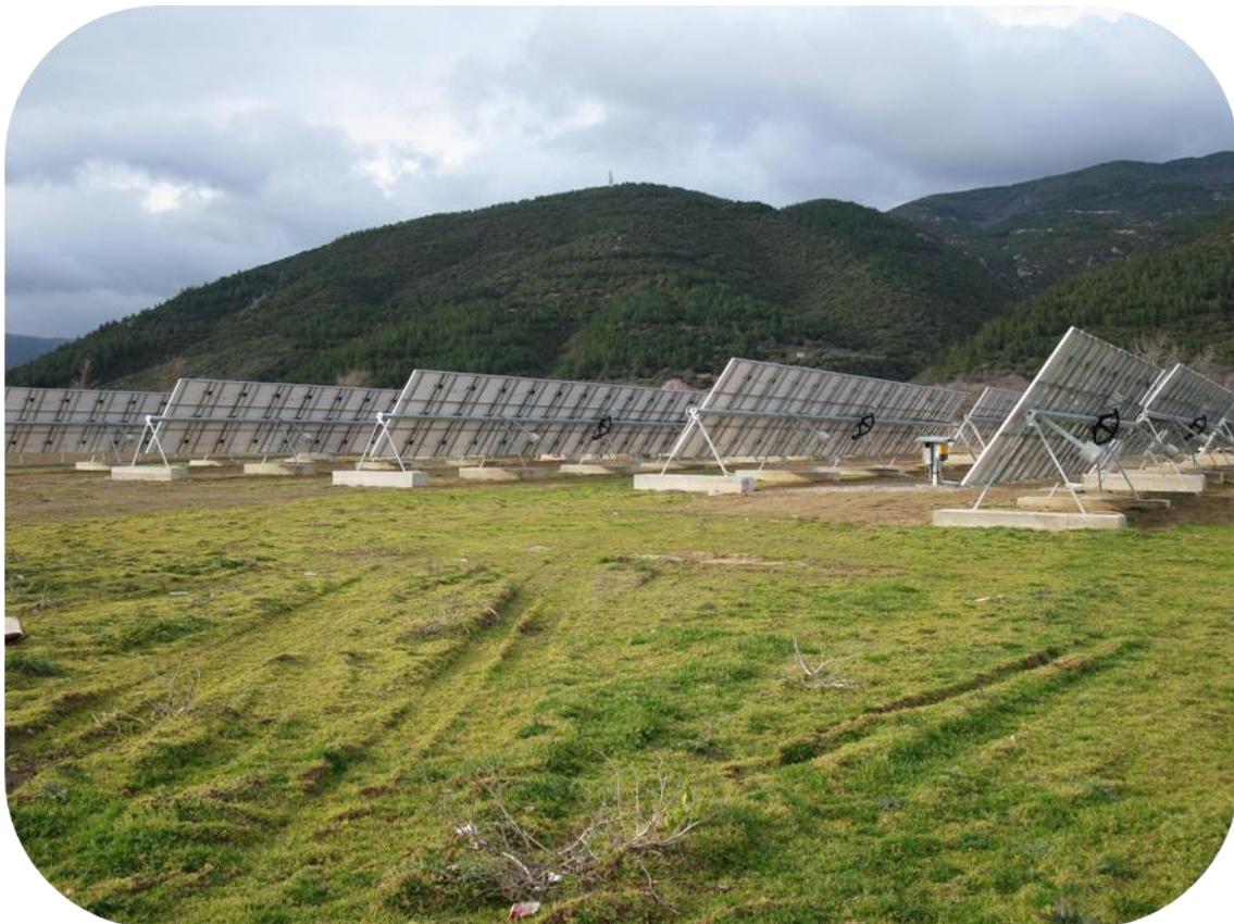
Solar plant In the north of Greece
